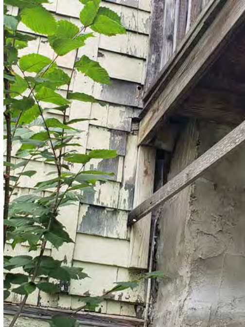
VIEW OF FAILING ENTRY DECK
