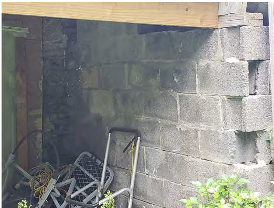
VIEW OF FAILING FOUNDATION SYSTEM
