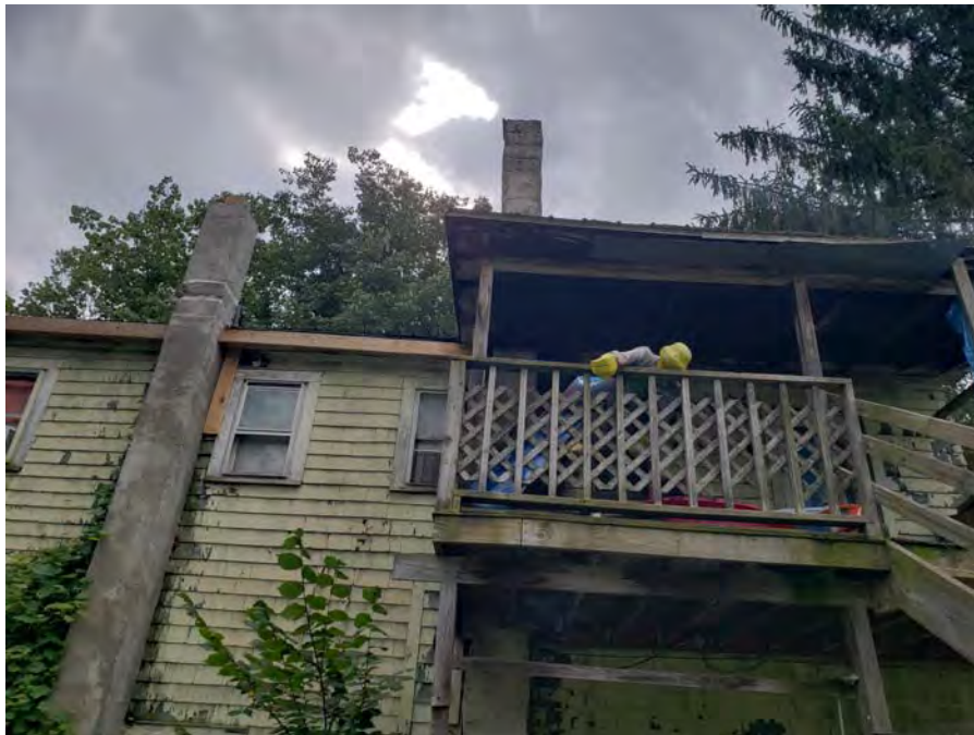
VIEW OF UNSTABLE CHIMNEYS
