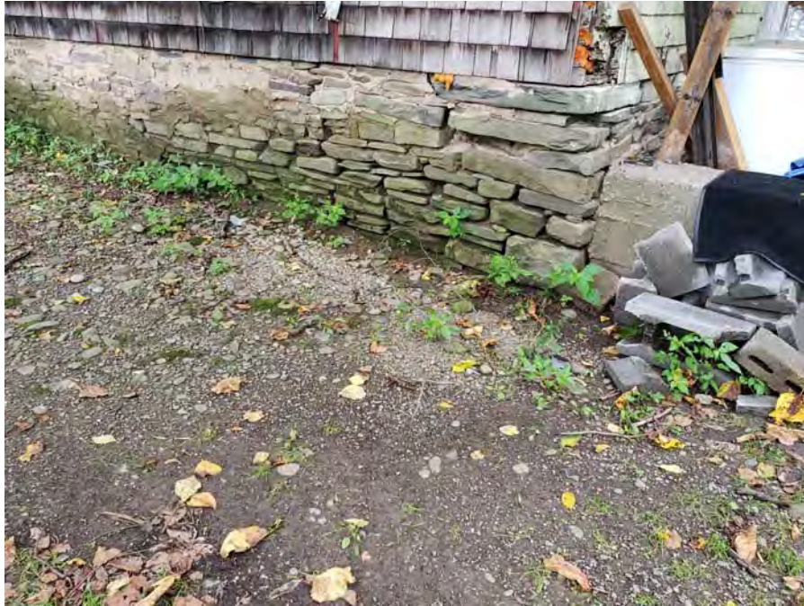
VIEW OF FAILING FOUNDATION SYSTEM
