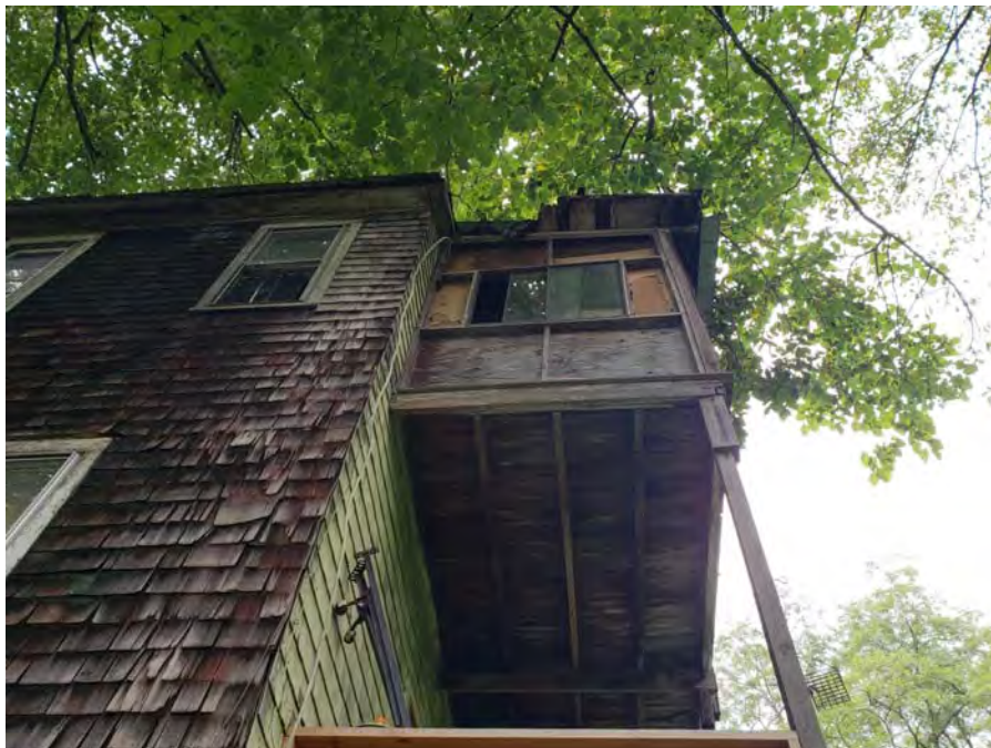
VIEW OF THE DETERIORATED ROOF SHEATHING, FASICA, & SOFFIT
