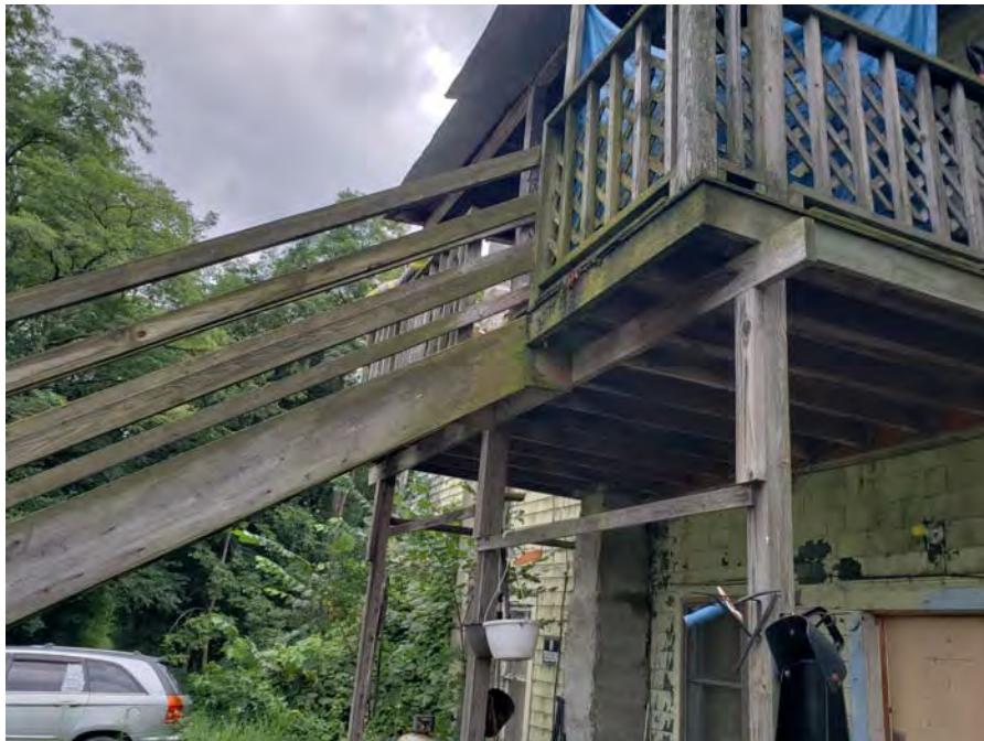
VIEW OF IMPROPERLY SECURED STAIRS
