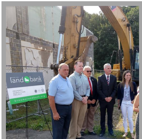
147-151 Front St., Town of Vestal pre-demolition press conference with County, Town and Land Bank Officials
